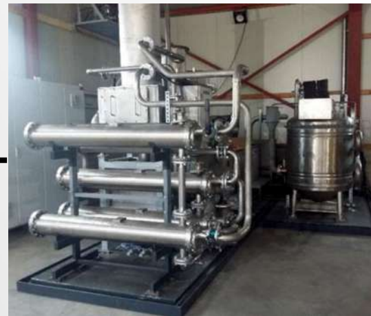
Wet gas cleaning unit
